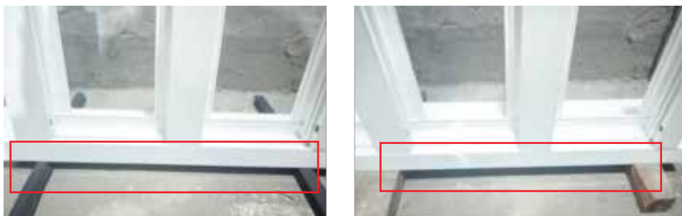
Image 12: The critical areas of fabricated window frame
