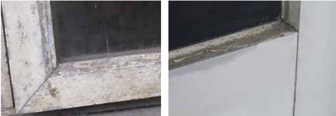
Image 20: Without proper maintenance in hazardous environment
