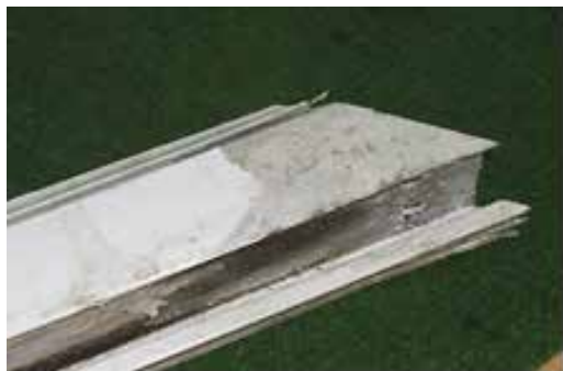
Image 13: Corrosion can crawl through corners
